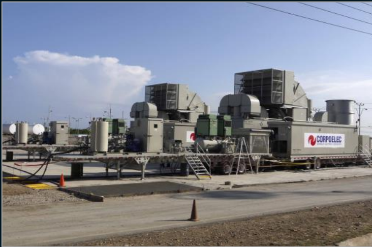
Turbinas a Gas
